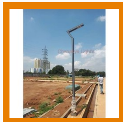
Steel Decorative Lighting Pole
