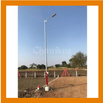
Street Light Pole
