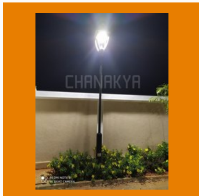
Postop Lighting Pole
